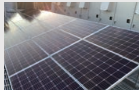
Solar panels installed at our headquarters
